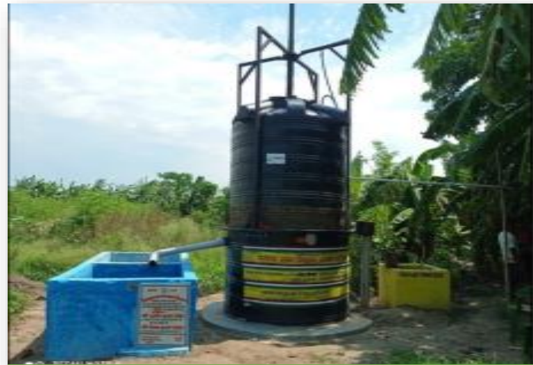
Sahaibganj- (Capacity-25 Cubic Mtr.)
